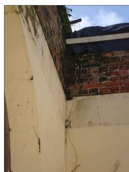
10 RACHADURA ENTRE AS PAREDES.
